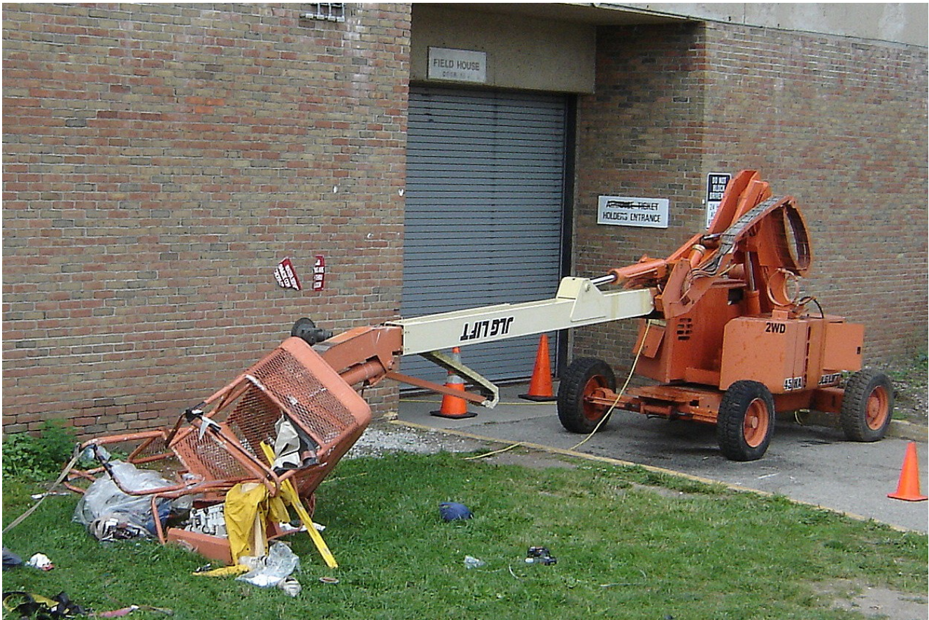
Photo 2. The aerial work platform collapsed during the incident and the lift basket crashed to the ground and landed on the grassy surface by the Field House (Photo courtesy of OSHA).
