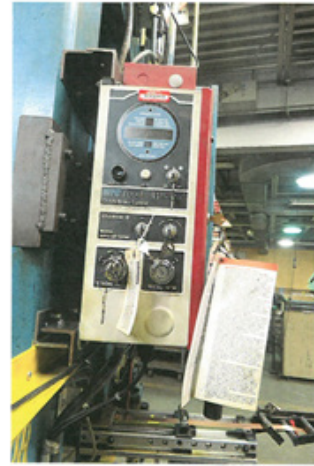
Photo 3: Key-required controller mounted to infeed side of press. (Photo courtesy of OSHA)
