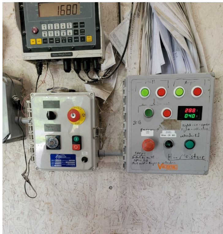
Photo 4. Unloader controls and emergency shutoff devices.
